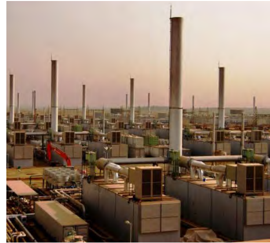
300 MW HFO Diesel Power Plant - IRAK
